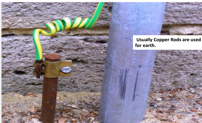
The size of the pipe used for earth is of 3.8cm diameter and 2.5m in length. More than 2 meters of the rod is buried in the 'earth pit'.
